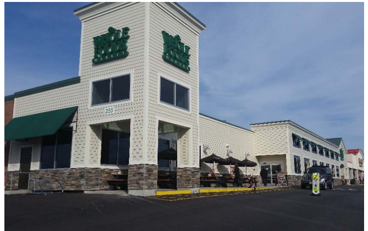
Over 10,000 sq. ft. of WrapShield SA Self-Adhered Water Resistive Vapor Permeable Air Barrier Sheet was installed on Whole Foods Market in Nashua, NH.
